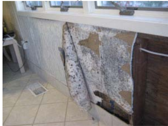
Building envelope moisture entry [Aldous 2008]
