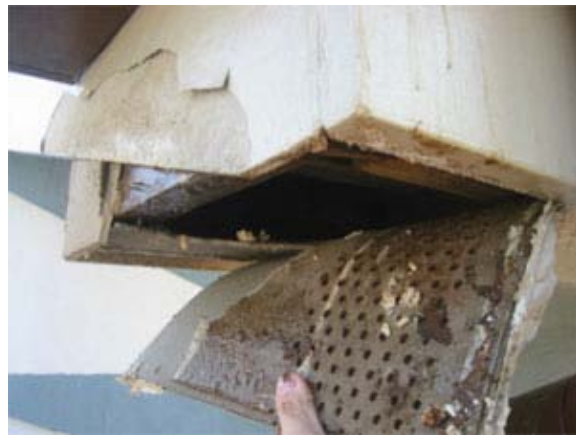
Building envelope moisture entry [Aldous 2008]
