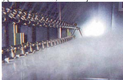
Active humidification downstream of a condensing cooling coil at cleanroom facility [Sellers no date]
