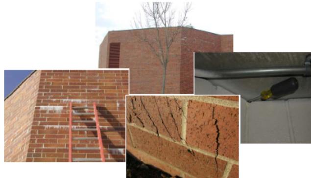
Damage to brick facade of pool building due to lack of specification for (a) sealing of air leakage paths in exterior envelope and (b) balancing to assure negative pressurization of pool area. Large newer middle school.
