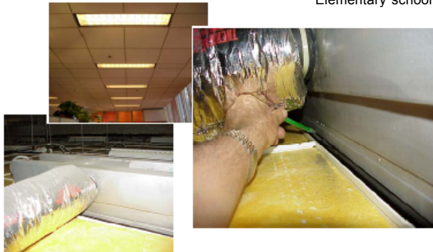
Inadequate cooling and excessive fan power consumption due to poor fit between light troffer diffusers and duct boot provided by a different supplier, allowing up to 25% of flow at diffuser to bypass directly into ceiling plenum. Highrise office tower.
